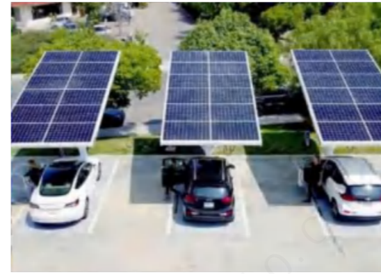
PV Storage & EV Charging
